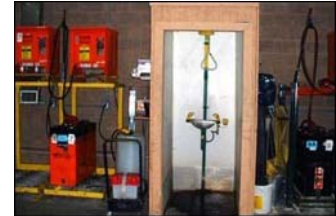
Figure 5. Large installations should have a plumbed drench shower and an eyewash.
