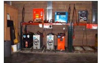
Figure 9. Battery charging area.
